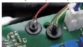
Example of probe with the double-sided tape
