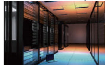
Data center thermal management
